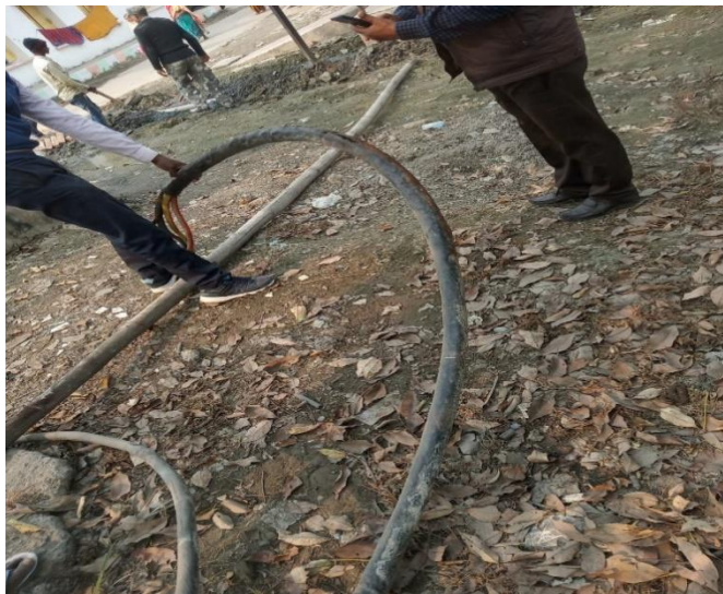
Figure 4: The electrical cable that got burnt at Sadar Hospital due to a short circuit caused by rainwater
