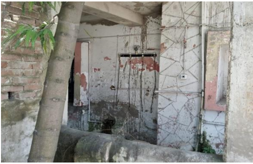
Figure 1: One of the five old manifolds at Sadar Hospital for two oxygen cylinders
