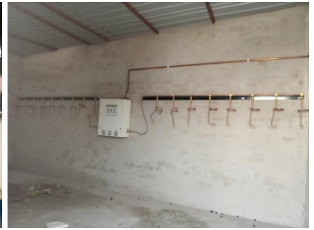
Figure 3: The new central manifold room at Sadar Hospital for eight cylinders
