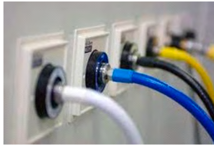
Figure 19: A set of medical gases outlets/inlets
