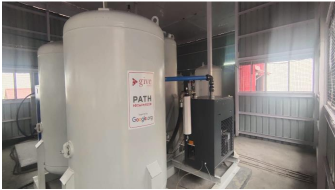
PSA plant supported by Google installed in the existing PSA shed by extending the area to accommodate an 800 liter per minute (LPM) plant
