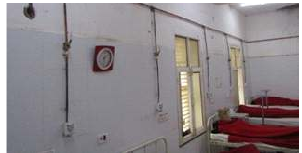
The MGPS setup in Central Jail Hospital
