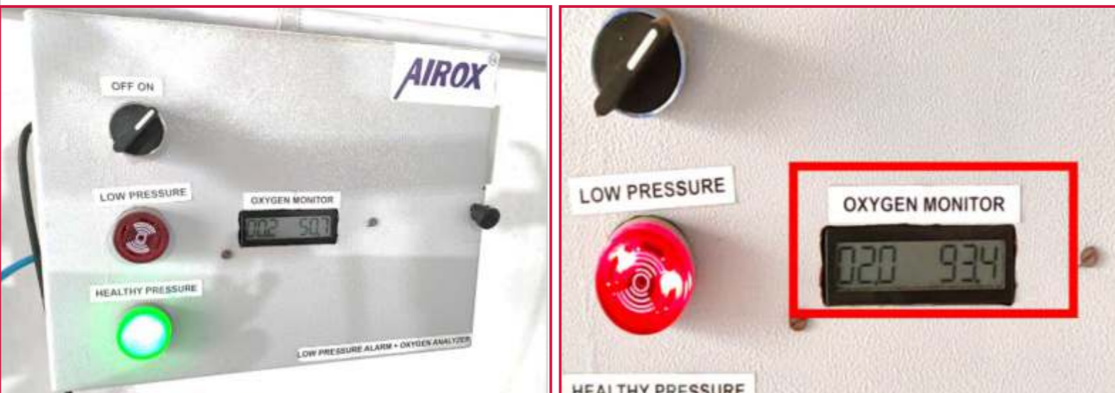
Image 2. Oxygen analyzer panel of the left showing oxygen pressure at 50.7 and on the right, after troubleshooting, showing 93.4
