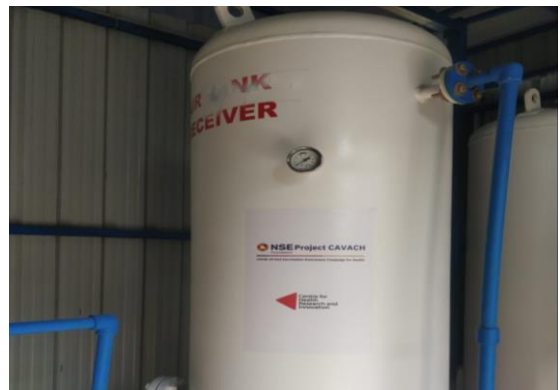
PSA plant of 200 LPM commissioned in CHC Kuchai
