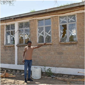
Derbew Abebaw points to broken health post windows damaged during conflict.
