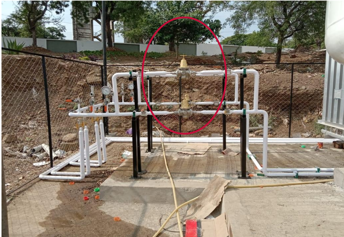
Figure 3: Two PRV connected to two vaporizers
