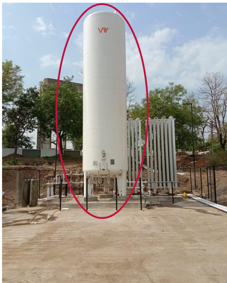
Figure 1: Liquid Medical Oxygen Tank
