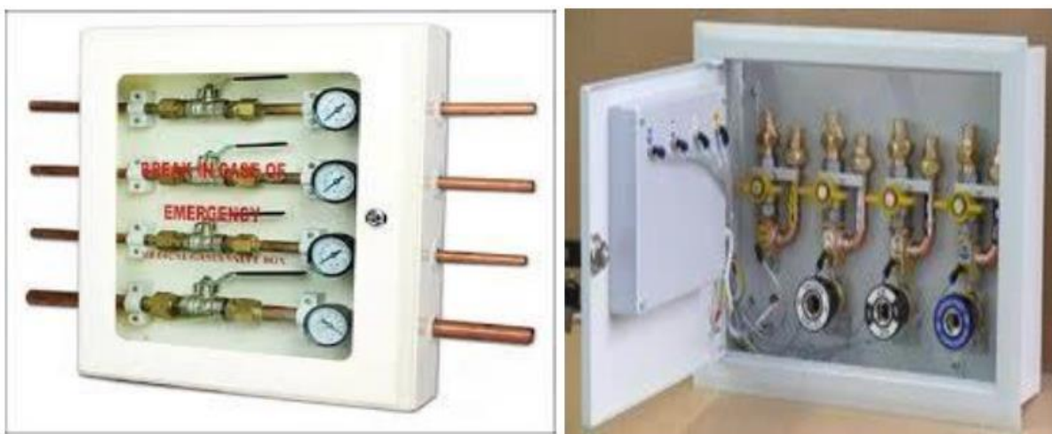
Figure 4: An Area Valve Service Unit
