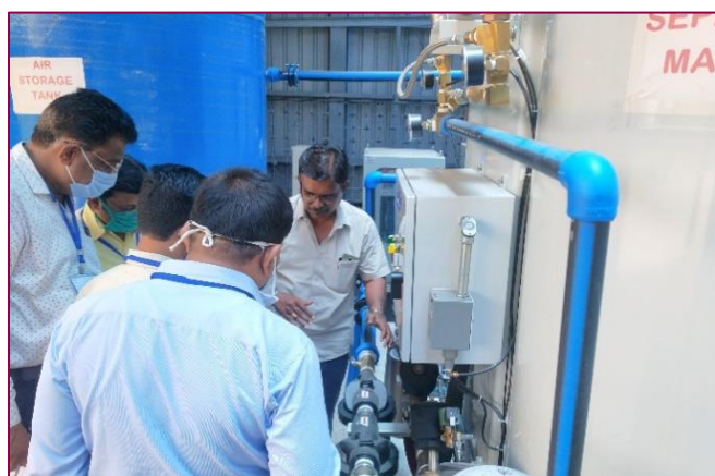
The expert trainer explaining about different components of a PSA oxygen generation plant in the hospital premises to the BME trainees
