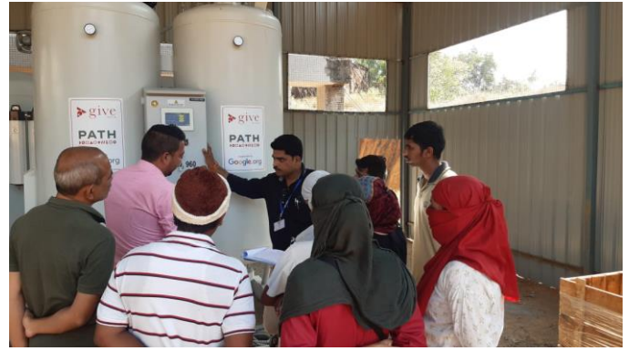
Figure 2: Training on PSA plant operations at Women's Hospital, Kudal, Sindhudurg district, Maharashtra, India
