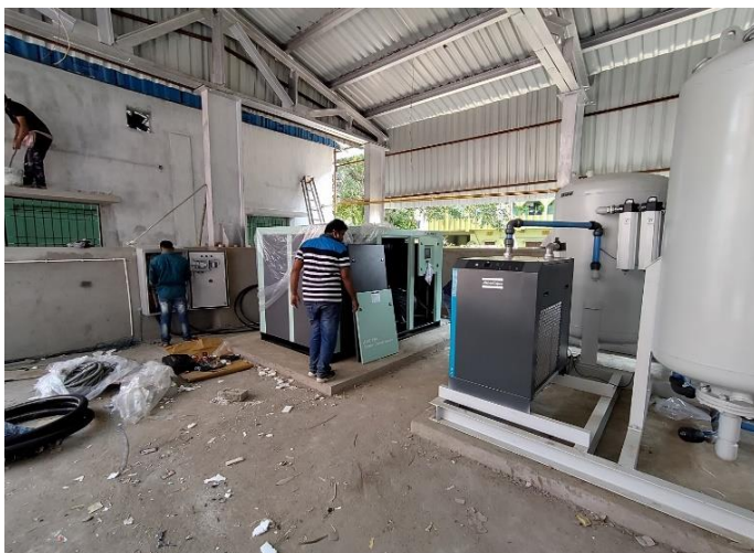
Installation and commissioning of PSA plant at DHH Keonjhar, Odisha, with the TASL team
