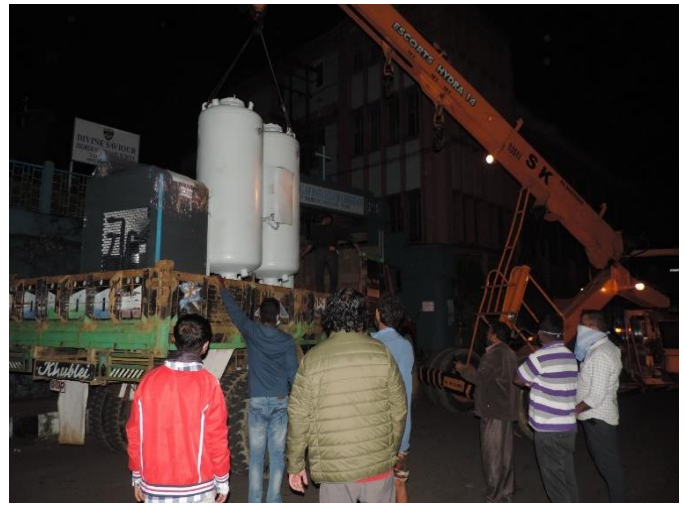
Unloading of the PSA plant at Nazareth Hospital, Meghalaya
